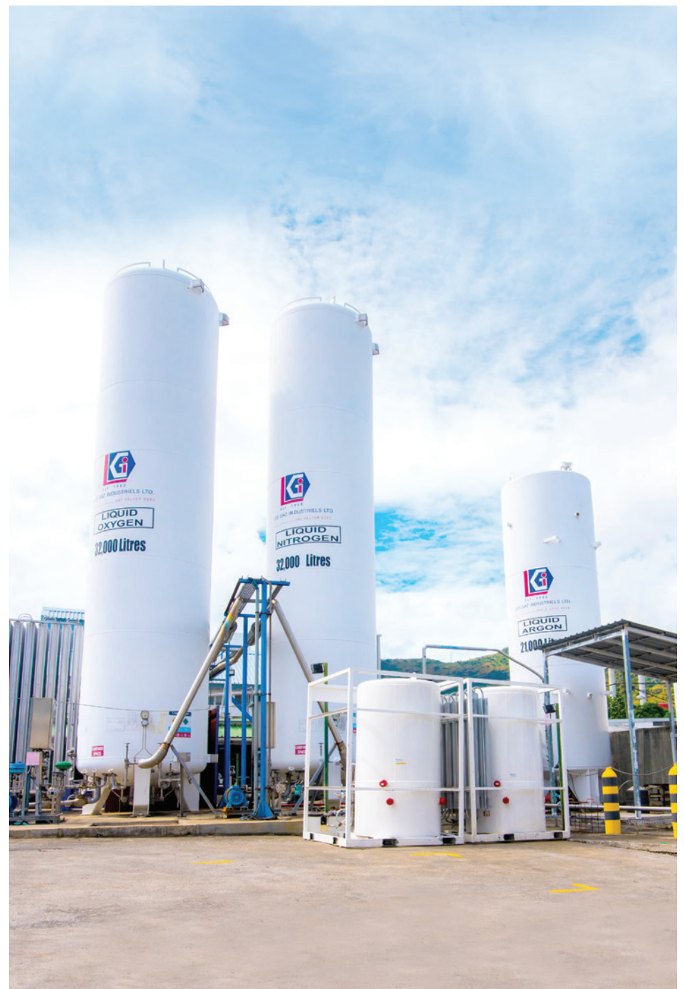
LGI's storage tanks for cryogenic oxygen, nitrogen and argon
